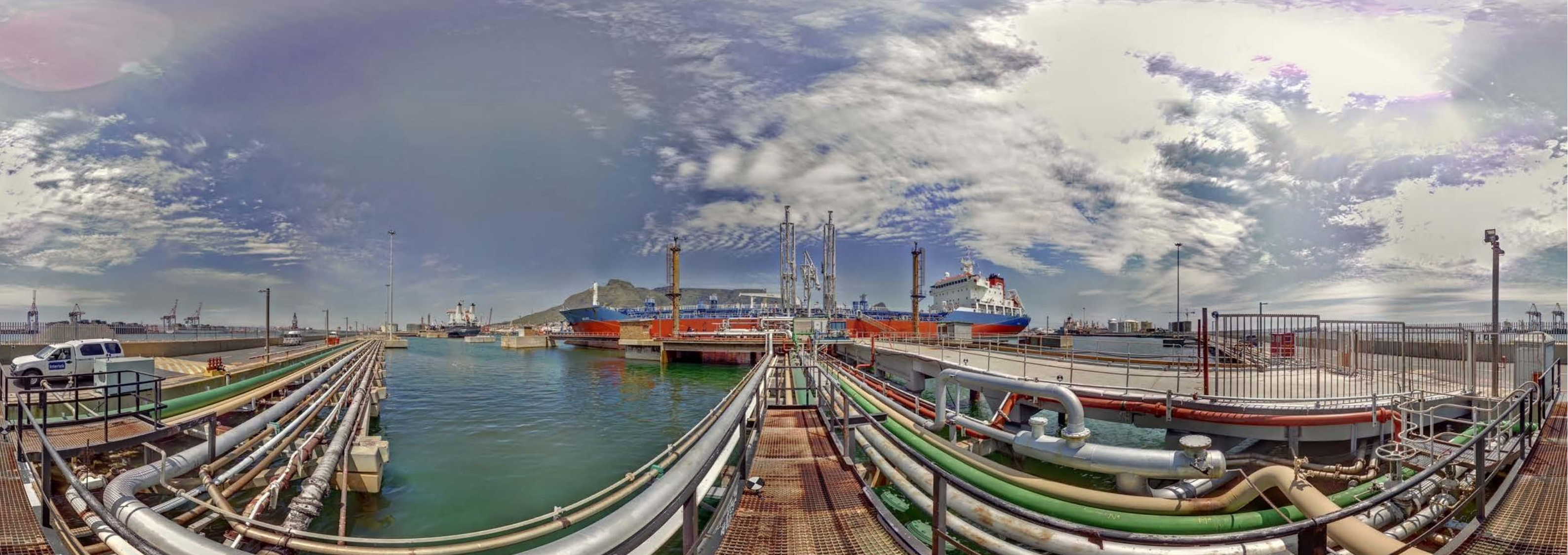
HDR point cloud of the Z+F IMAGER® 5010C in the harbour of Cape Town, South Africa. The colour of the pipes indicate their content and condition. Source: Satmap Solutions/HORTS Solutions, South Africa
